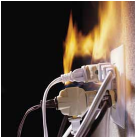
Each year home electrical fires claim nearly 500 lives, injure more than 2,000 and cause nearly a billion dollars in property losses.
