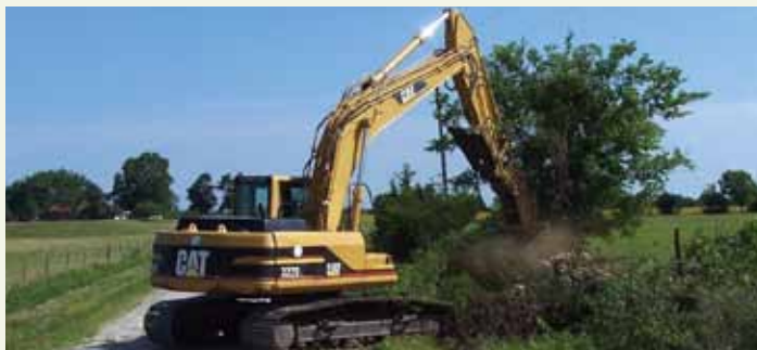
1 Operator Jodie Zwahlen with Zwahlen Dozing operates a 322B Caterpillar trackhoe with a tree saw to eliminate line clearance problems.
