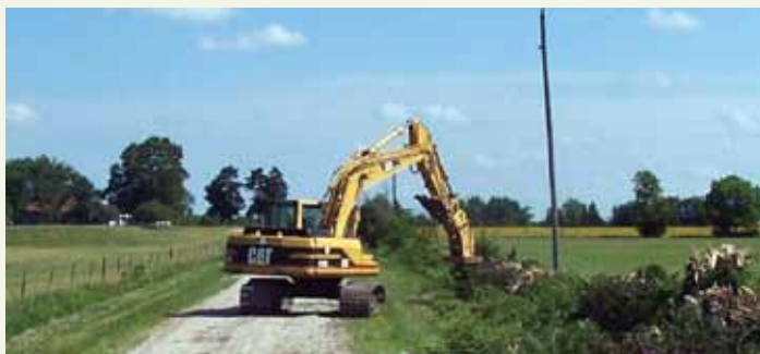
3 The line was cleared of excess vegetation within 15 minutes and ready to replace.
