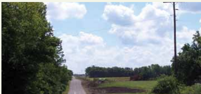
4 All vegetation has been removed from the right-of-way. This stretch of line is ready to be replaced.
