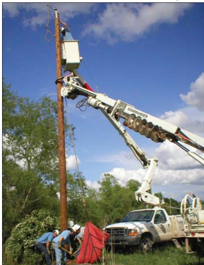
Twin Valley linemen Tyler Kennett, in bucket, Kenny Cole, Joe Brooks, Tom Shelton and John Hibbs, on the ground, repair the lines after a spring storm.
